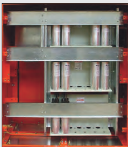
Capacitor Load Bank accessed via rear door of assembly.
