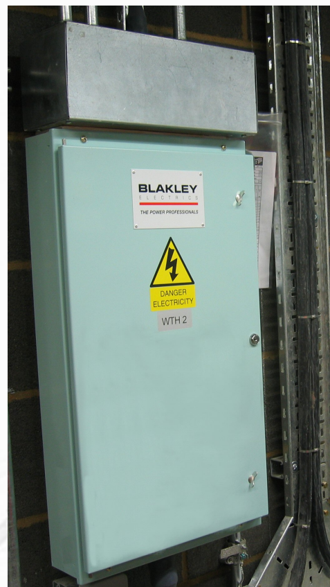
8W TP Board in Section 12 Installation
