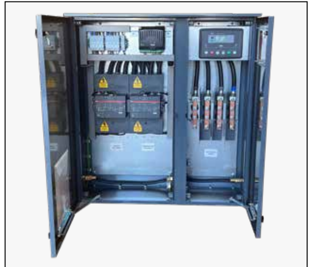
500A Automatic Mains Failure Panel
