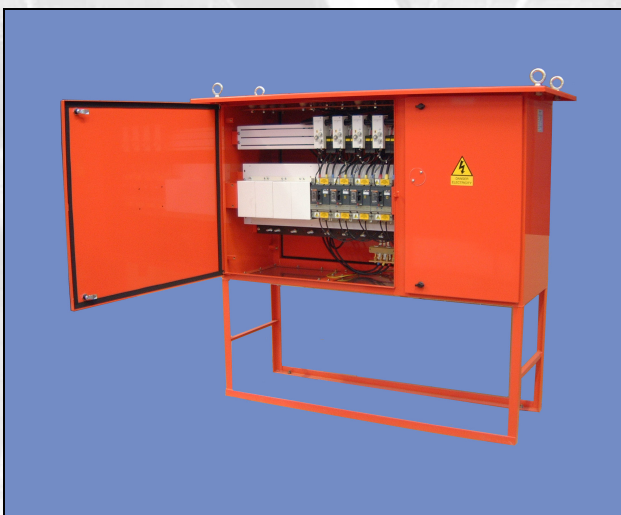
S140285 800A MDA with shield plates removed
