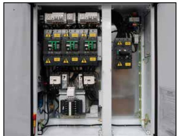
A7085396 - Doors open and Internal IPXXB Shield Plates Removed
