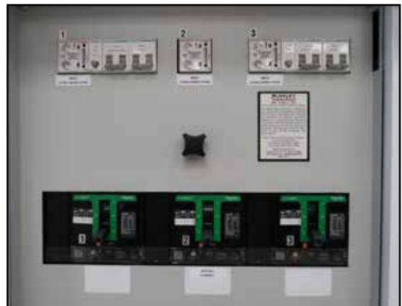
Distribution Door Open Showing MCCBs, MRCDs and Switches for Diode Reversal and ECM By-pass
