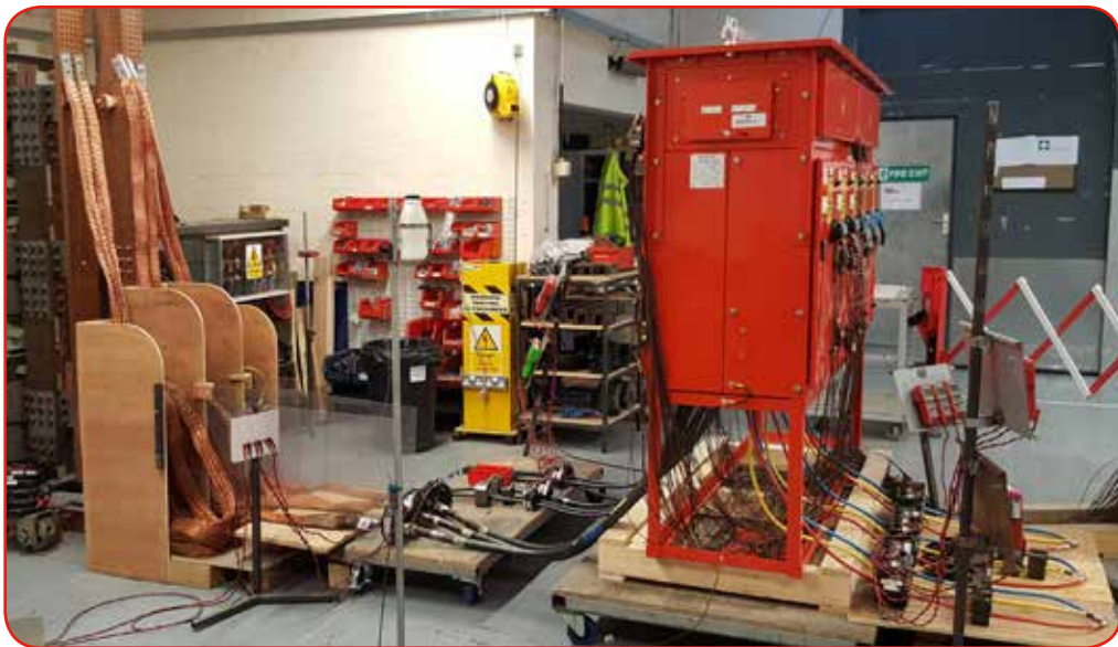
400A Form 4 Type 3 Mains Distribution Assembly undergoing temperature rise testing at a third party, UKAS approved, test laboratory.
