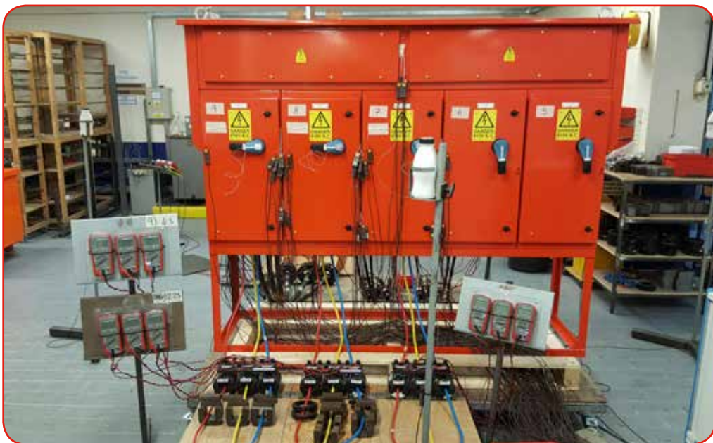
The testing, which was conducted over a period of 3 days, established the overall full load rating of the IP55, non-vented, Mains Distribution Assembly, as well as a rating for each of the Fuse Combination Switches, with nominal ratings ranging from 100A to 400A.
