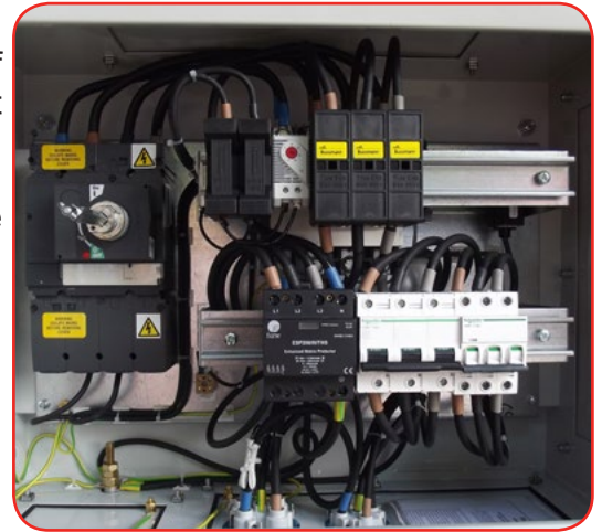
Three-phase Type 1 Protector supplied via 63A HRC fuses
