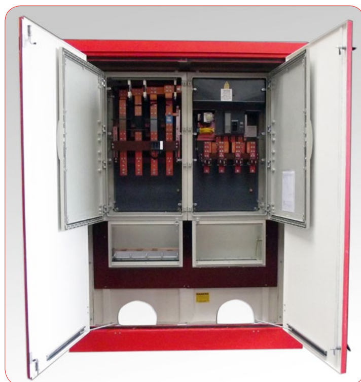
1250A Combined CTC & RCD, SSE specification, Housed in an S050473 ISIA GRP Cabinet
