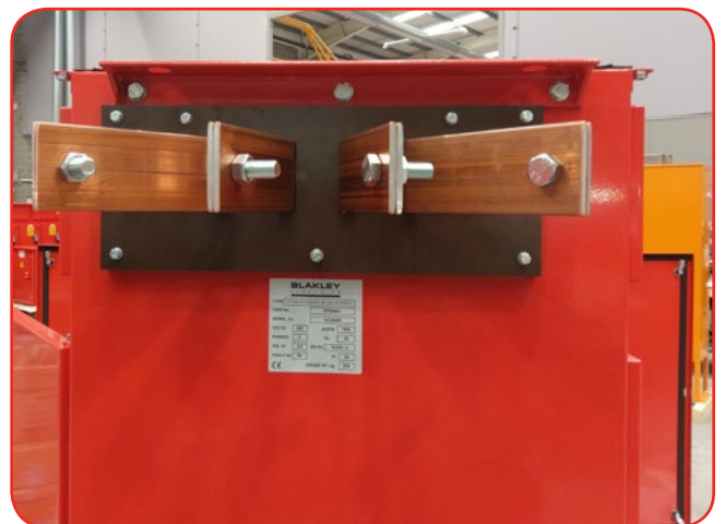
Connections for testing bus bar system
