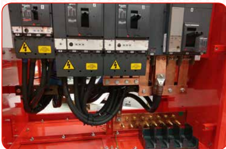
Connections for testing outgoing MCCB / RCDs
