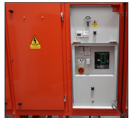
Distribution compartment with hinged inset panel lowered.
