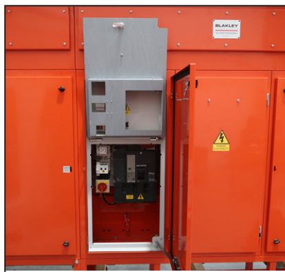
Distribution compartment with hinged inset panel raised.
