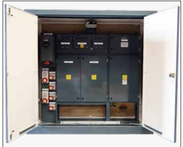
DSU part no. A7293182 comprising of an IP55 stainless steel enclosure mounted within a heavy duty GRP outer enclosure.
