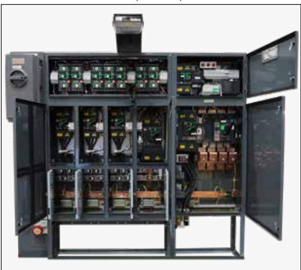
Inner switchboard of DSU part no. A7293182 prior to outer GRP enclosure being fitted. All shield plates removed.
