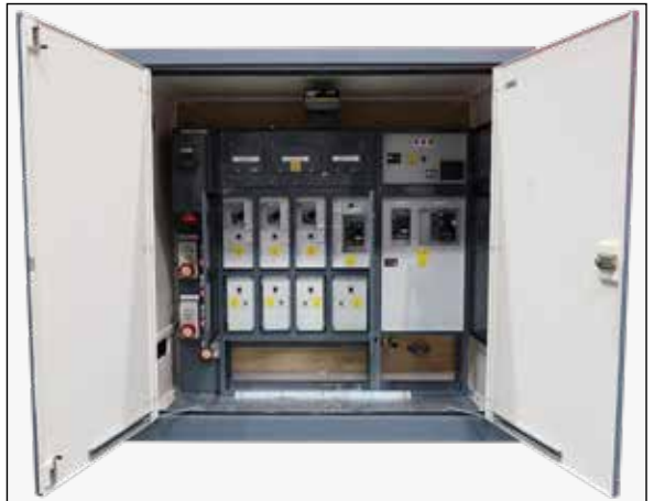
DSU part no. A7293182, switchboard doors open, all shield plates in place.
