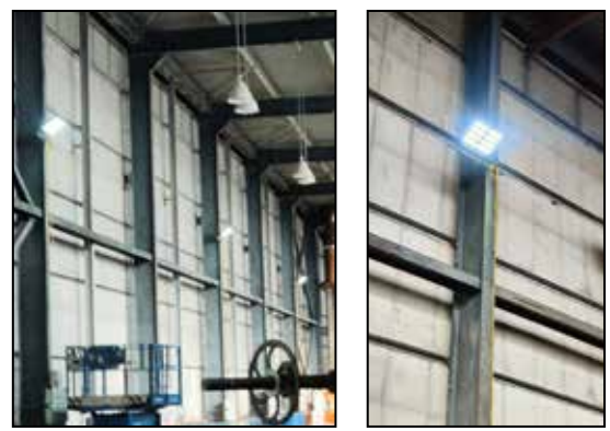
Ultra 450W floodlights are installed at high level and supplied via 110V flexible cable.
