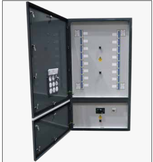
A7293373 Distribution Board with 250A 4P incoming switch and 16 no. 40A 4P / 30mA DC Immune MRCDs.
