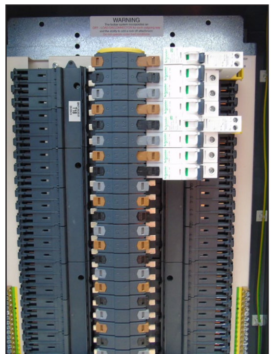
A7292676 - RCBOs with Plug On Neutral fitted alongside standard MCBs
