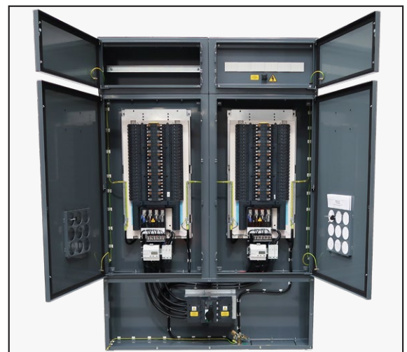
A7292704 - Multi-Section MCB Board with shield plates removed. Pans individually metered.
