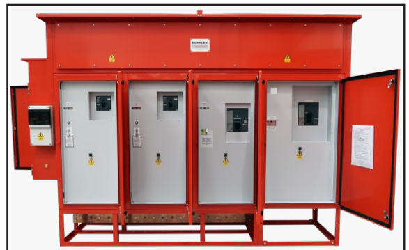
A7191759 Form 4 MDA 1600A, Separate Stand Extension Supplied for Fitting On Site
