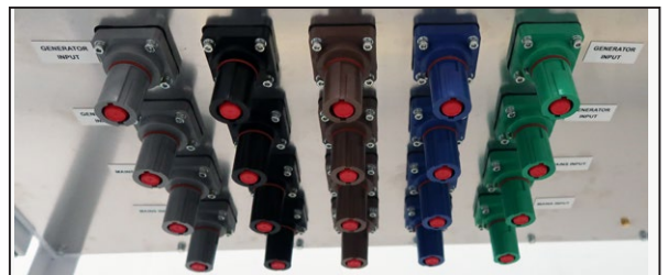
Incoming single pole connectors, 2 no. per phase, neutral and earth, mains & generator
