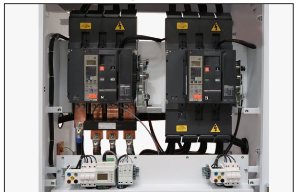
Incoming auto changeover arrangement, shield plate removed
