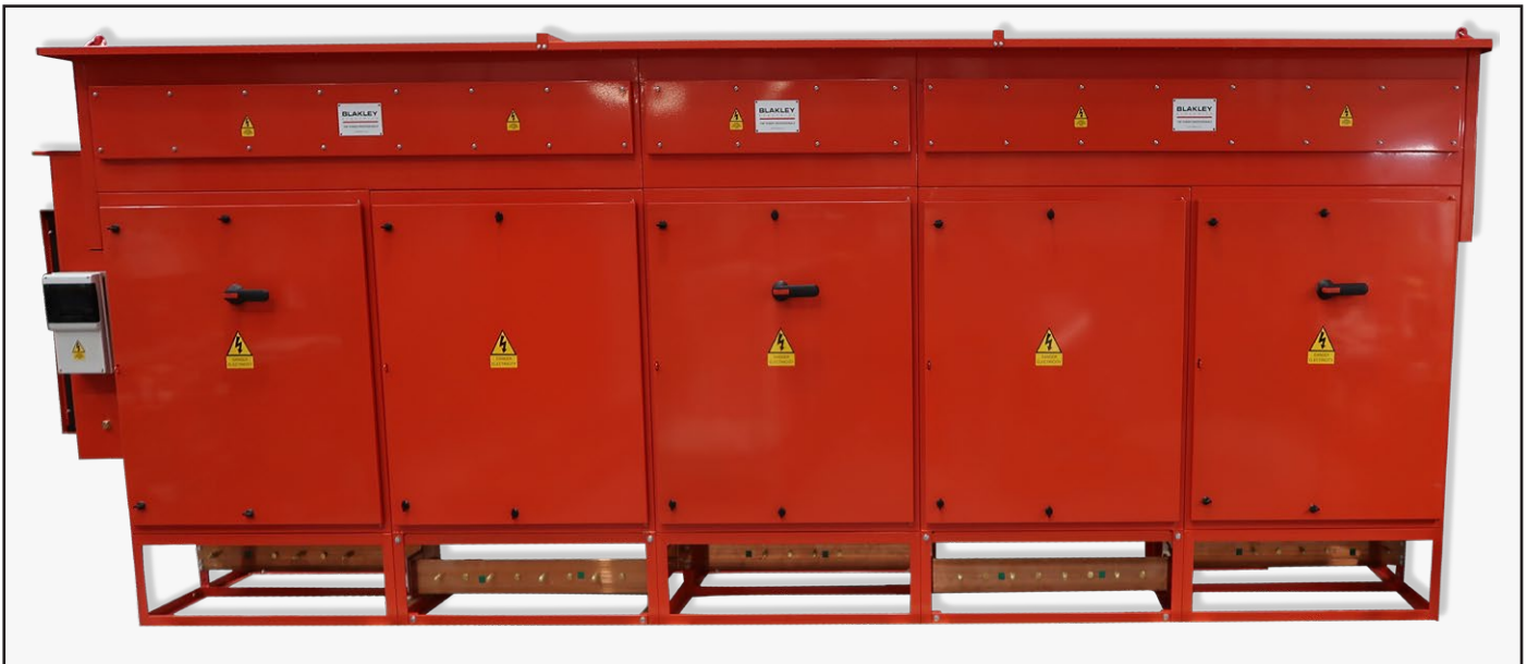
Generator Interface / Distribution Assembly with 6 x 800A Incomers and 2 x 3200A Outgoing ACBs, part number A7193399
