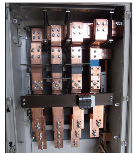
A7085196 CT chamber with termination arrangement to receive a total of 11 no. incoming cables
