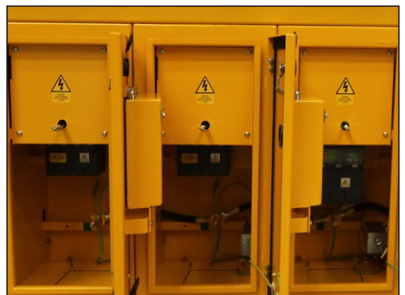
Each functional unit is housed in its own compartment, fully segregated from the bus bars.
