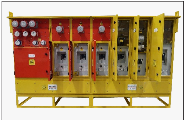
A7292950 Subway Dockside Service Unit, 630A, Rear View with Hard Wired and Plug-in Outlets
