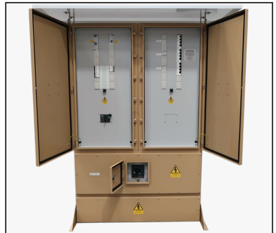
A7293069 4P 400A main switch with 12 way MCB pan assembly and 3 x 100A MCB/MRCD outgoing ways.
