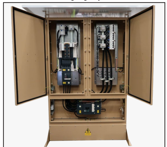
Assembly also incorporates anti-condensation heaters
